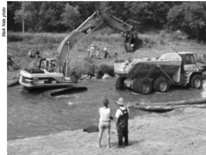
Clearwater Conservancy project grant manager Katie Ombolski (foreground left) and Trout Unlimited volunteer Bob Carline (right) look on as limestone is unloaded by a trackhoe and used to secure a log deflector on Spring Creek. Other TU volunteers rest on the bank until it is safe to reenter the stream.
